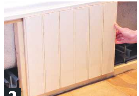
3 Attach remaining buttons to frame. Position panel and press against marker points to give indents
